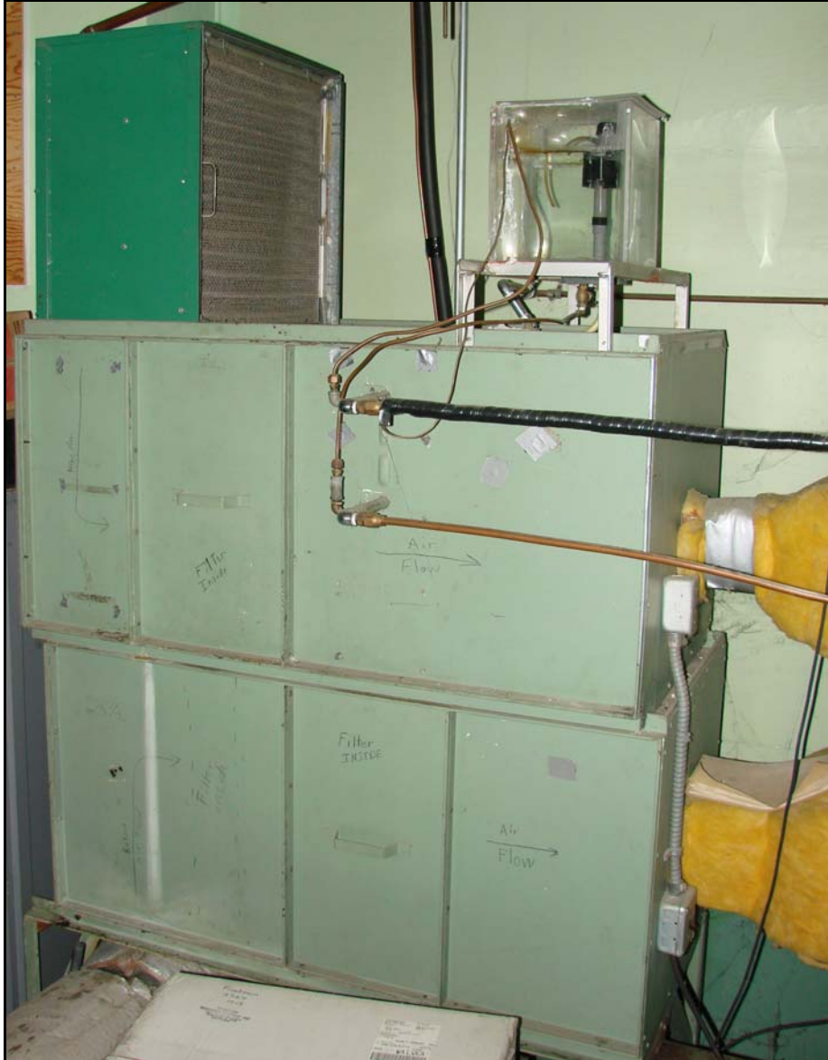
Air filtering and tempering system for the Coude' camera room. It also provides a positive pressure to the room to help prevent dust infiltration.
