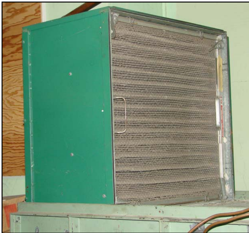
This is the air makeup intake in need of changing.
